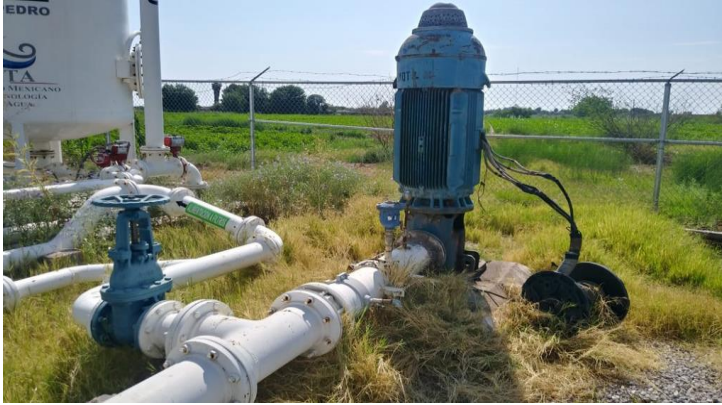
Brackish water well
